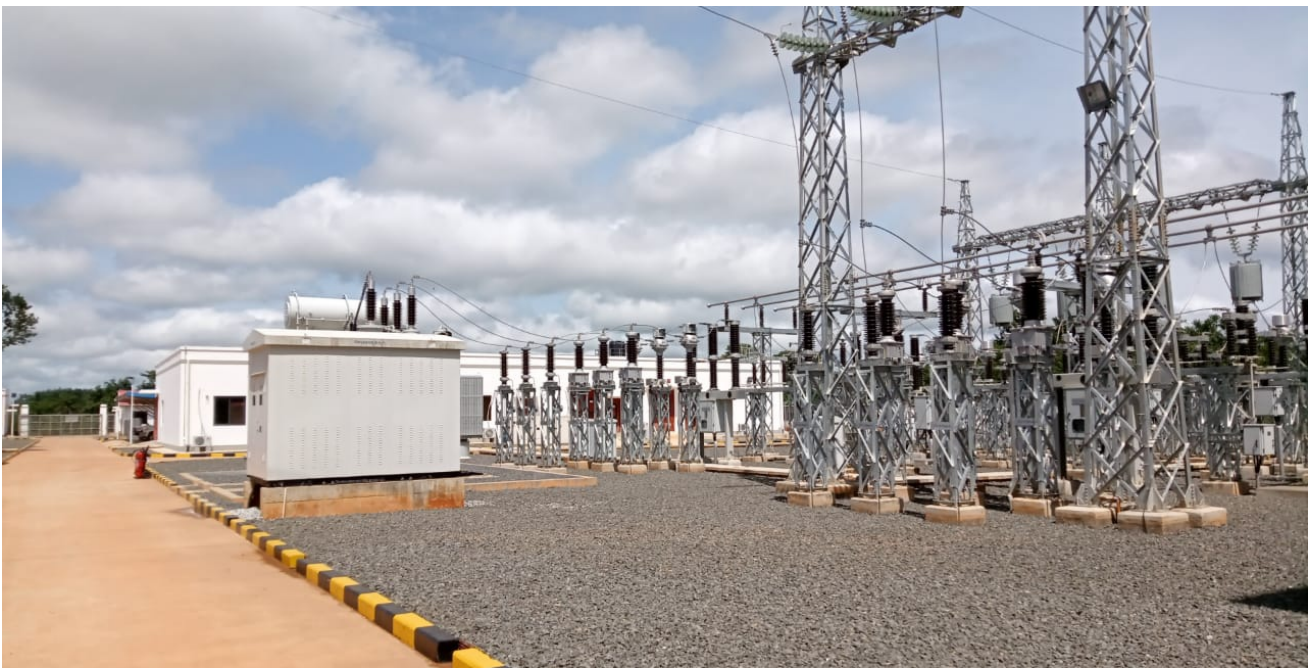
TRANSCO CLSG Botota Substation in Bong County
